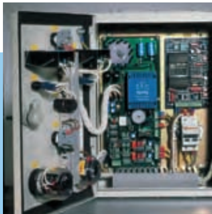
Control box with printed circuits and selector switch for digital read out.
